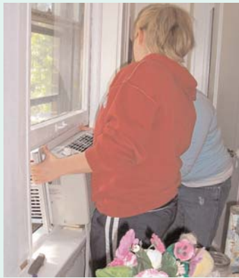
Service providers install an air conditioner in the home of an EnergyCare client.
